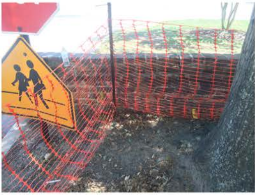
(1), Greene Street - Campus Elevation Partial height wall with major vertical crack.
