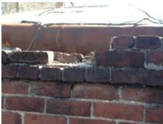
Missing Bricks in Coping on Sumter
