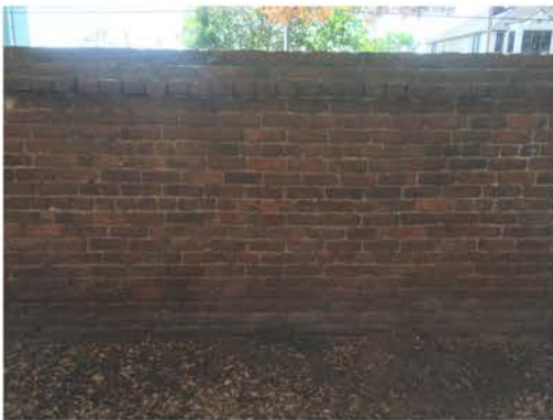
(250), Sumter Street - Campus Elevation Full height wall. Multiple repointing required.
