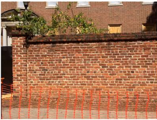
(61), Sumter Street - Street Elevation Full height wall with pier. Multiple brick face cracking.
