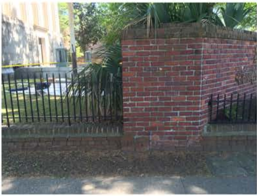
(157), Pendleton Street - Street Elevation Large diagonal corner wall with small partial height wall and fence.. Mortar and cap replacement required. Multiple repointing and brick repair required.
