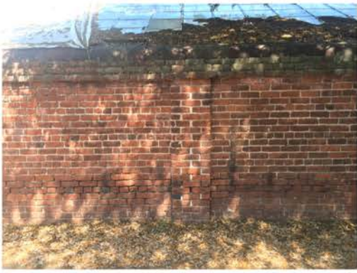
(73), Sumter Street - Street Elevation Full height wall with single pier. Multiple mortar and repointing issues. Vegetation issues at cap.
