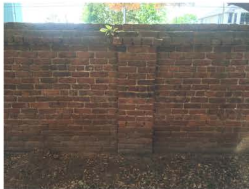
(251), Sumter Street - Campus Elevation Full height wall with pier. Multiple repointing required. Vegetation issues.
