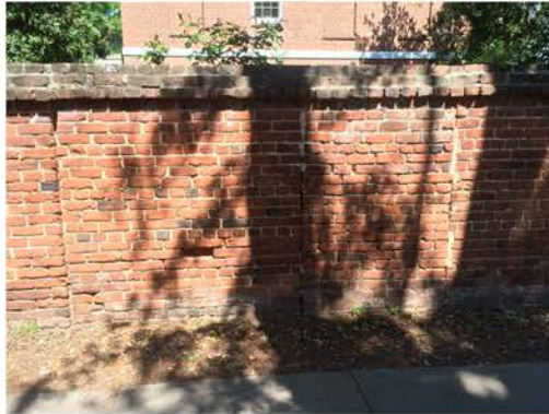
(80), Sumter Street - Street Elevation Full height wall with single pier. Large portion of the wall needs replacing. Bricks missing.
