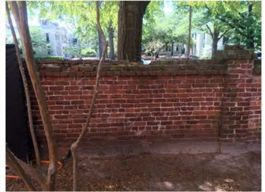
(30), Sumter Street - Campus Elevation Full height wall. Cap repair required.
