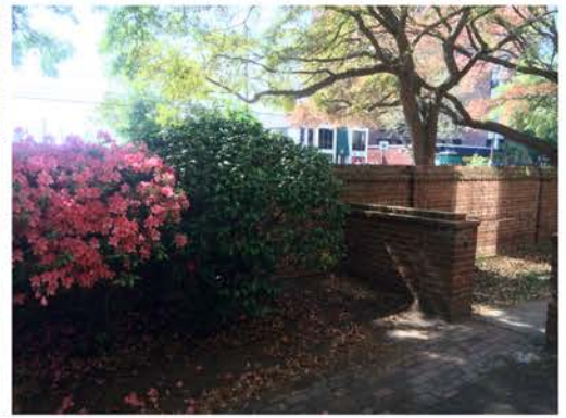
(243), Sumter Street - Campus Elevation Full height wall to partial height wall. Multiple repointing required.
