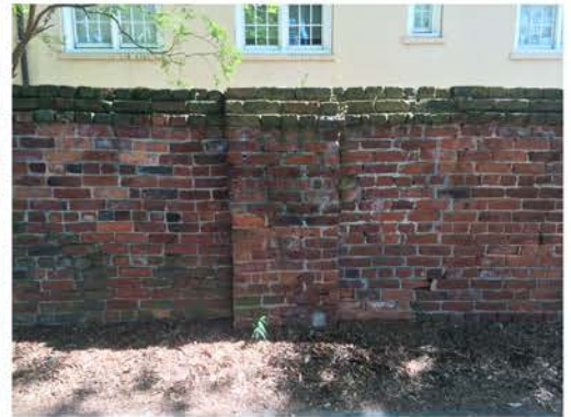
(201), Pendleton Street - Street Elevation Full height wall with pier. Multiple mortar repointing required.
