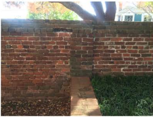
(253), Sumter Street - Campus Elevation Full height wall with adjacent partial height wall. Multiple repointing required. Cap work required.
