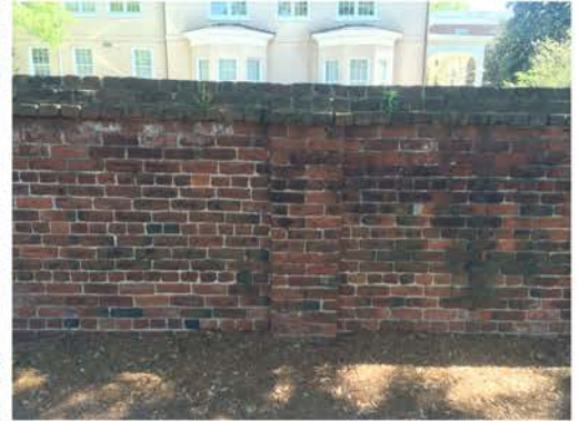
(186), Pendleton Street - Street Elevation Full height wall with pier. Cap and vegetation issues.
