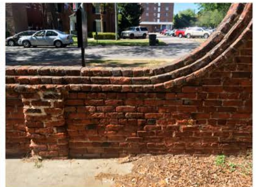
(300), Pendleton Street - Campus Elevation Partial wall height to full height wall. Repeating required. Multiple mortars.
