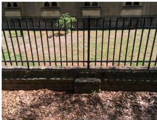
(167), Pendleton Street - Street Elevation Low wall with fence and pier. Multiple repointing issues.
