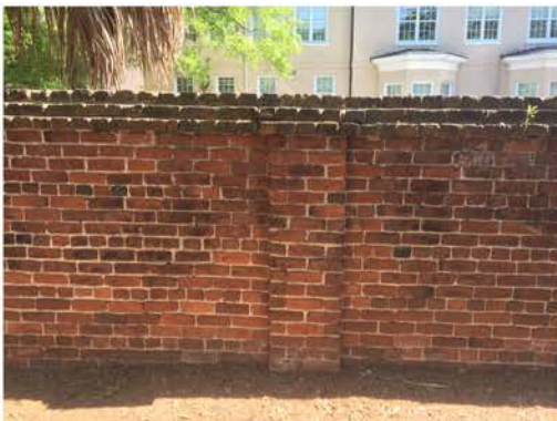
(190), Pendleton Street - Street Elevation Full height wall with pier. Cap and vegetation issues. Multiple mortar repointing required.
