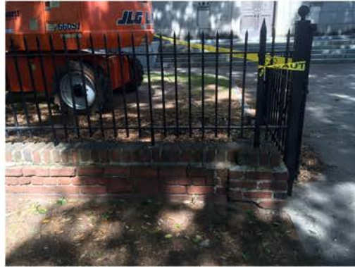
(149), Sumter Street - Street Elevation Low wall with fence and gate. Mortar and cap replacement required.
