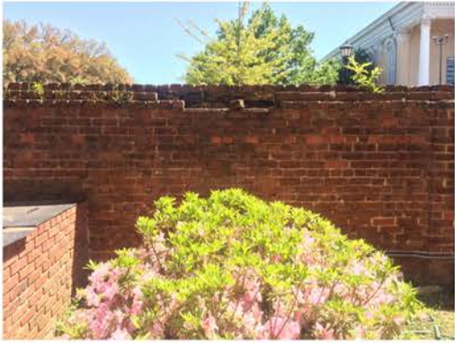
(10), Greene Street - Campus Elevation Full height wall. Cap replacement and repair required.
