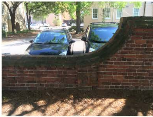
(194), Pendleton Street - Street Elevation Full height to partial height wall with pier. Multiple mortar repointing required.
