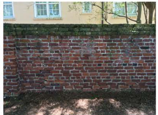
(204), Pendleton Street - Street Elevation Full height wall. Multiple mortar repointing required. Cap replacement. Vegetation issues.
