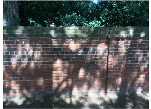
(138), Sumter Street - Street Elevation Partial height wall with small pier. Incorrect mortar replacement.
