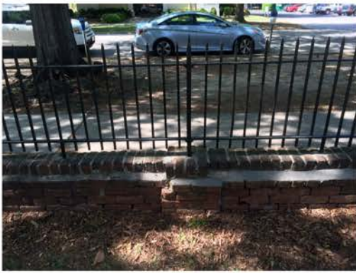
(277), Pendleton Street - Campus Elevation Low wall with fence. Multiple repointing issues. Cap mortar issue.
