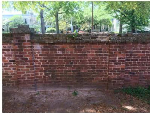
(32), Sumter Street - Campus Elevation Full height wall. Cap repair required. Remove vegetation.
