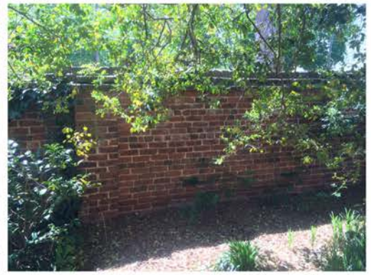
(87), Sumter Street - Campus Elevation Full height wall. Cap repair required.
