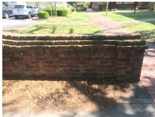
(179), Pendleton Street - Street Elevation Low wall requiring brick and mortar replacement.
