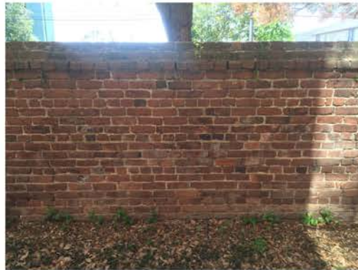
(248), Sumter Street - Campus Elevation Full height wall. Multiple repointing required. Vegetation issues.
