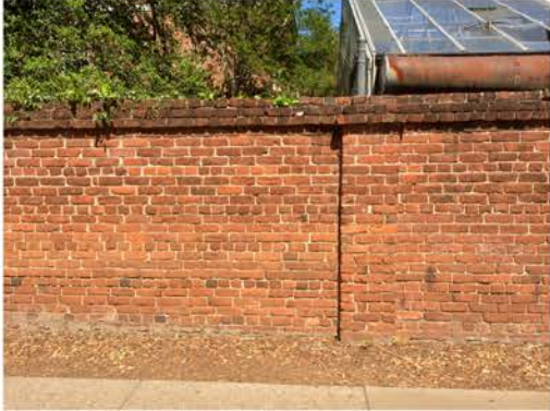
(76), Sumter Street - Street Elevation Full height wall with single pier. Multiple mortar and repointing issues. Vegetation issues at cap.
