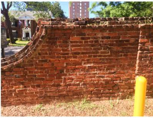
(301), Pendleton Street - Campus Elevation Full wall height with multiple structural issues. Repointing required. Multiple mortars.
