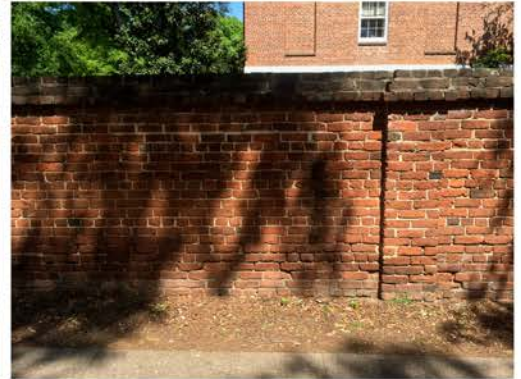
(81), Sumter Street - Street Elevation Full height wall with single pier. Base missing mortar.
