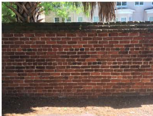
(191), Pendleton Street - Street Elevation Full height wall with pier. Cap and vegetation issues. Multiple mortar repointing required.
