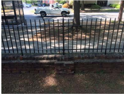
(269), Pendleton Street - Campus Elevation Low wall with fence and pier. Multiple repointing issues. Vegetation issues. Cap mortar issue.
