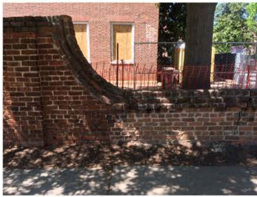
(38), Greene Street - Street Elevation Partial height wall with major vertical crack. Transition to full height wall.
