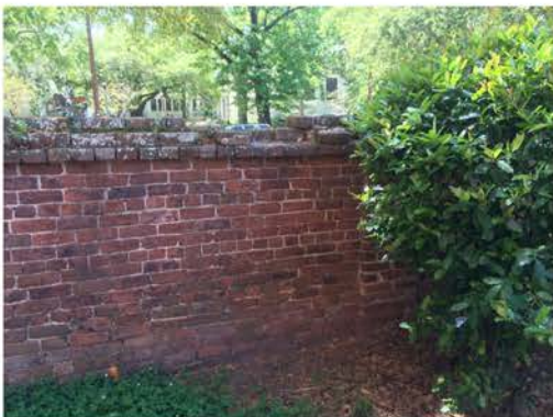
(34), Sumter Street - Campus Elevation Full height wall and adjacent wall. Cap repair required.
