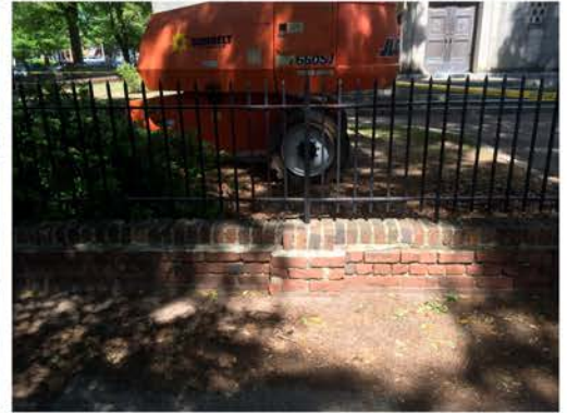
(150), Sumter Street - Street Elevation Low wall with fence and pier. Mortar and cap replacement required.
