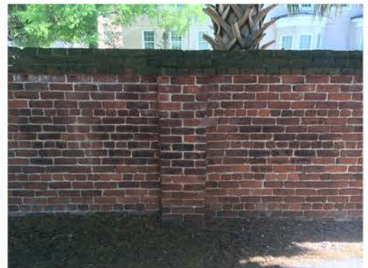
(192), Pendleton Street - Street Elevation Full height wall with pier. Cap and vegetation issues. Multiple mortar repointing required.
