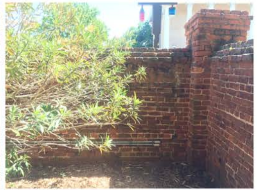
(15), Greene/Sumter Street - Campus Elevation - Corner Full height wall. Repointing and vegetation removal required. Existing conduit removal required. Major vertical crack at large pier.
