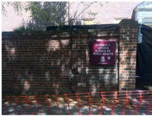
(62), Sumter Street - Street Elevation Full height wall with two piers. Major repair to small pier.
