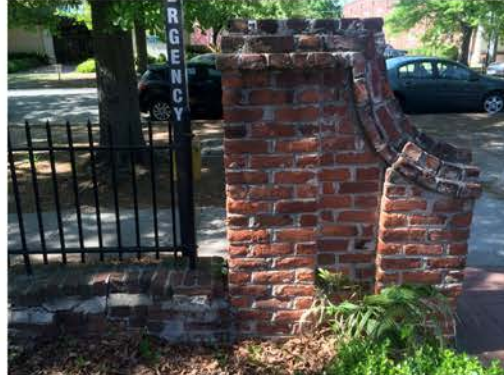
(281), Pendleton Street - Campus Elevation Double pier with gate. Repointing required.
