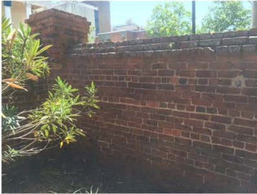
(16), Sumter Street - Campus Elevation Full height wall. Repointing required.
