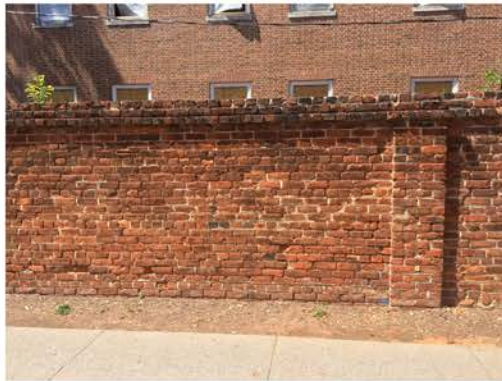
(44), Greene Street - Street Elevation Full height wall. Missing brick.
