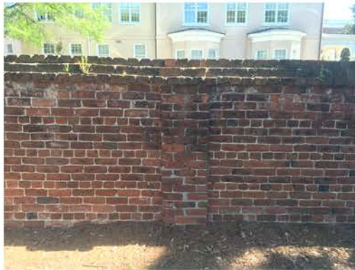
(188), Pendleton Street - Street Elevation Full height wall with pier. Cap and vegetation issues.
