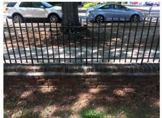
(276), Pendleton Street - Campus Elevation Low wall with fence. Multiple repointing issues. Cap mortar issue.
