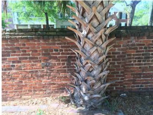
(293), Pendleton Street - Campus Elevation Full height wall with pier. Repointing required. Multiple mortars. Tree too close to wall.
