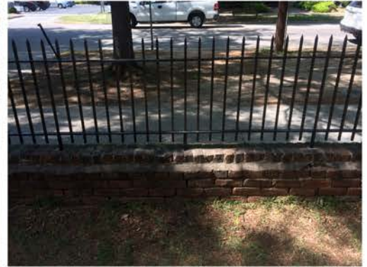
(270), Pendleton Street - Campus Elevation Low wall with fence. Multiple repointing issues. Vegetation issues. Cap mortar issue.
