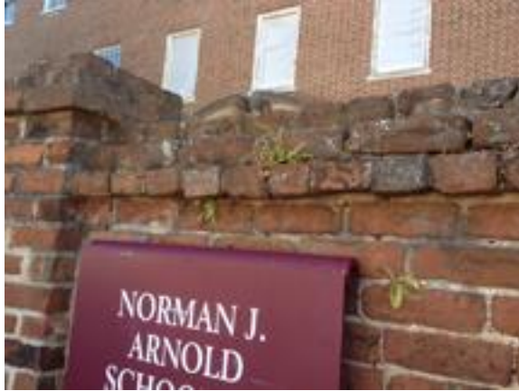
Top Course of Wall by Sumter near Greene (Note mortar recession and vegetation in coping courses.)
