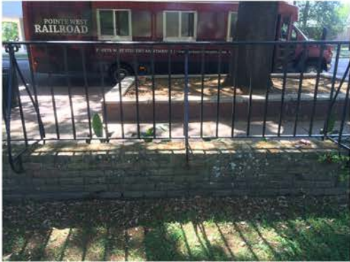
(232), Sumter Street - Campus Elevation Partial height wall with vertical rail. Vegetation issues typ.
