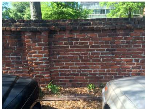
(287), Pendleton Street - Campus Elevation Full height wall with pier. Repointing required. Vegetation issues. Multiple mortars.
