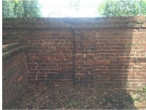
(245), Sumter Street - Campus Elevation Full height wall to partial height wall with pier. Multiple repointing required.
