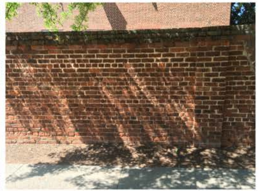
(39), Greene Street - Street Elevation Full height wall. Vegetation issues.
