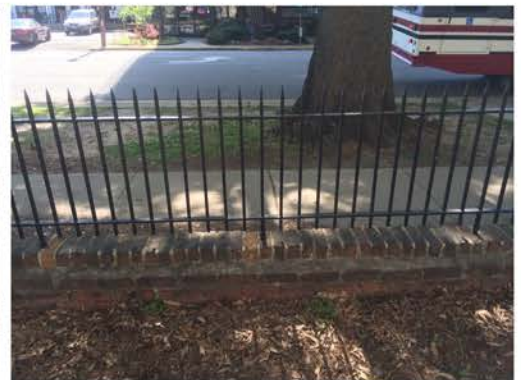
(264), Sumter Street - Campus Elevation Partial height wall with metal fence. Multiple repointing required. Cap work required. Metal to mortar connection needs work.
