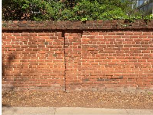
(77), Sumter Street - Street Elevation Full height wall with single pier. Multiple mortar and repointing issues. Cap repair required..
