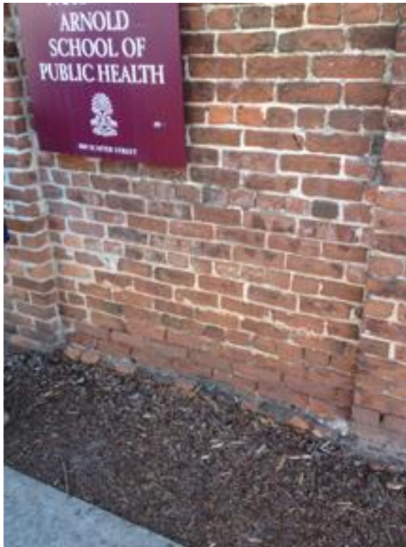
Lower Courses of Wall by Sumter near Greene (Note mortar recession in lower wall.)
