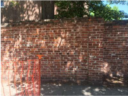
(52), Sumter Street - Street Elevation Full height wall. Brick bump out. Multiple repointing issues.
