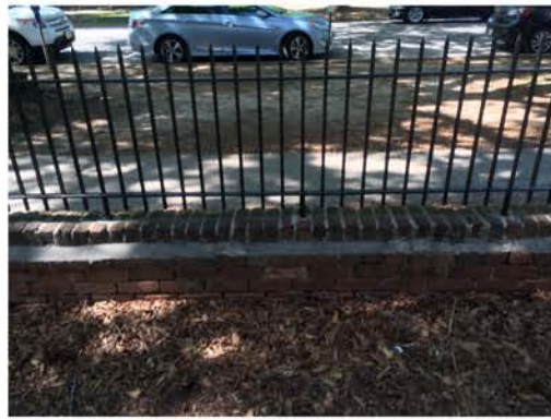
(278), Pendleton Street - Campus Elevation Low wall with fence. Multiple repointing issues. Cap mortar issue.
