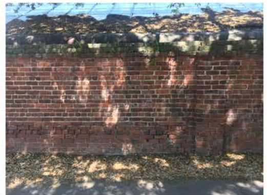
(72), Sumter Street - Street Elevation Full height wall with single pier. Multiple mortar and repointing issues.
