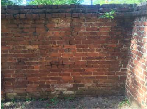
(316), Pendleton Street - Campus Elevation Full wall height. Major repointing required. Multiple mortars.
