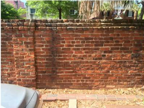
(292), Pendleton Street - Campus Elevation Full height wall with pier. Repointing required. Multiple mortars. Vertical cracking.
