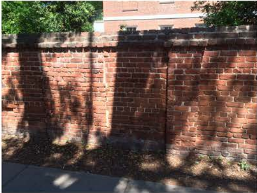
(79), Sumter Street - Street Elevation Full height wall with single pier. Large portion of the wall needs replacing.
