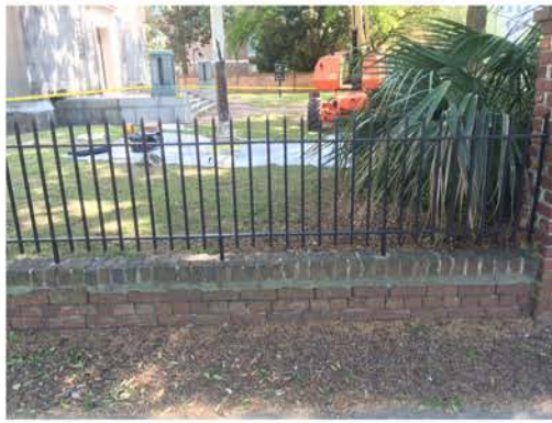
(158), Pendleton Street - Street Elevation Low wall with fence and pier. Mortar and cap replacement required.
