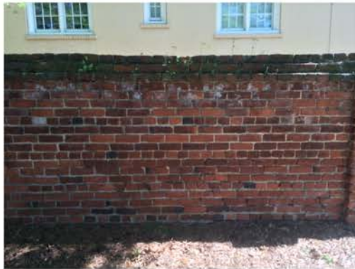
(200), Pendleton Street - Street Elevation Full height wall. Multiple mortar repointing required. Vegetation required.
