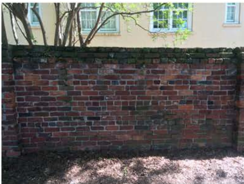
(202), Pendleton Street - Street Elevation Full height wall with pier. Multiple repointing required.
