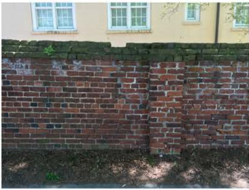
(205), Pendleton Street - Street Elevation Full height wall with pier. Multiple mortar repointing required. Cap replacement. Vegetation issues.
