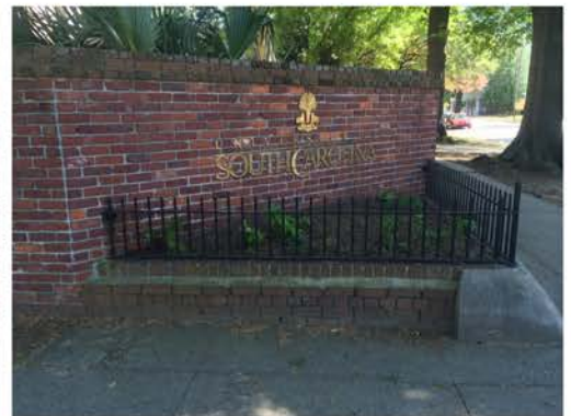
(156), Pendleton Street - Street Elevation Large diagonal corner wall with small partial height wall and fence.. Mortar and cap replacement required. Multiple repointing and brick repair required.
