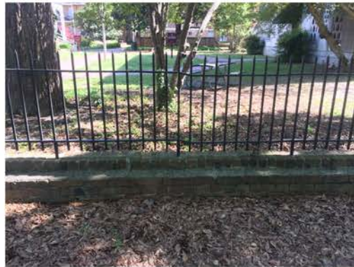
(176), Pendleton Street - Street Elevation Low wall with fence. Multiple repointing issues.
