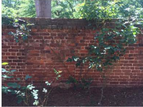
(89), Sumter Street - Campus Elevation Full height wall. Multiple vertical cracks.
