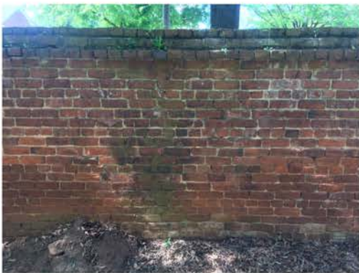
(310), Pendleton Street - Campus Elevation Full wall height. Major repointing required. Multiple mortars.
