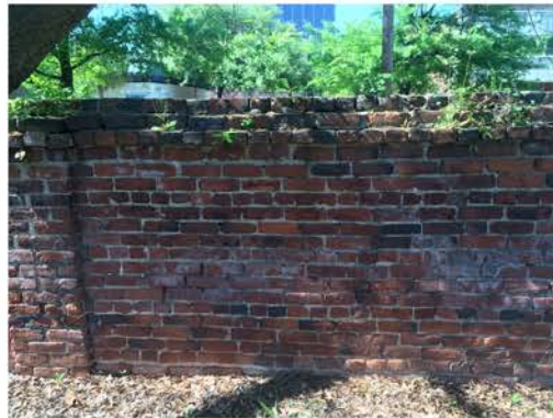
(284), Pendleton Street - Campus Elevation Full height wall with pier. Repointing required. Vegetation issues.
