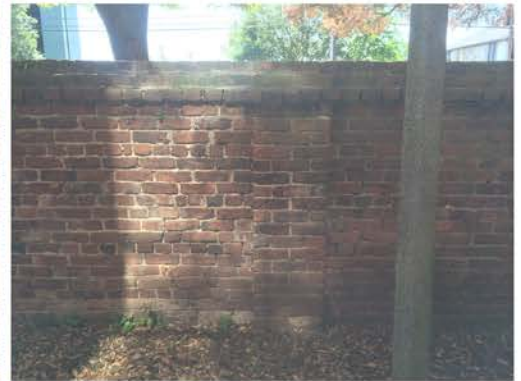
(249), Sumter Street - Campus Elevation Full height wall with pier. Multiple repointing required. Pole adjacent.
