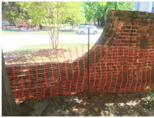
(2), Greene Street - Campus Elevation Partial height wall to full height wall transition.
