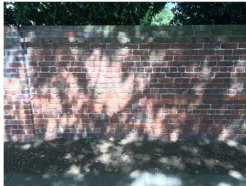
(140), Sumter Street - Street Elevation Full height wall with small pier. Multiple mortar replacement.
