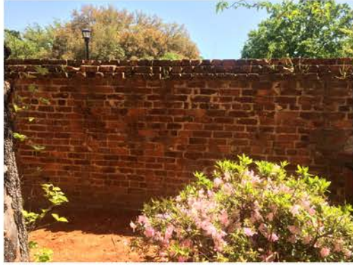
(8), Greene Street - Campus Elevation Full height wall. Minor cap replacement and repair required.
