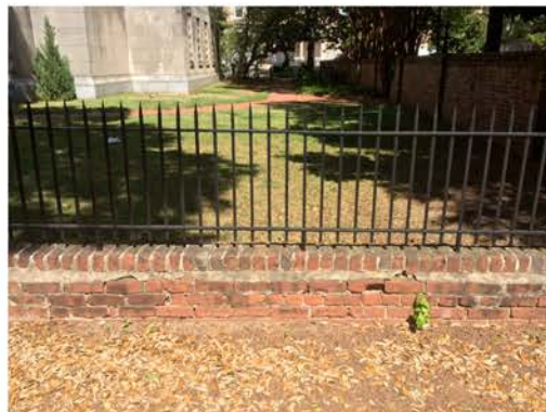
(143), Sumter Street - Street Elevation Low wall with fence. Brick repair/replacement required. Mortar replacement required.
