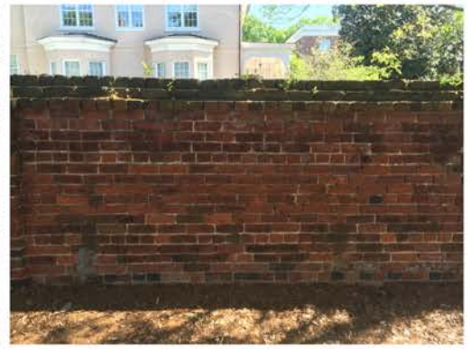
(183), Pendleton Street - Street Elevation Full height wall with pier. Cap and vegetation issues.
