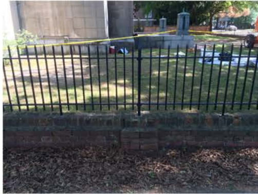
(161), Pendleton Street - Street Elevation Low wall with fence and pier. Multiple repointing issues.
