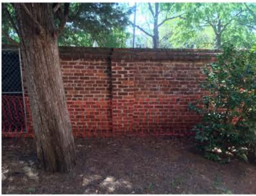
(25), Sumter Street - Campus Elevation Full height wall. Cedar tree close to wall.
