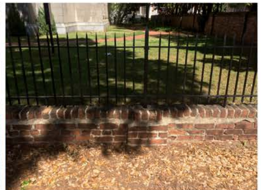
(144), Sumter Street - Street Elevation Low wall with fence. Mortar and cap replacement required.
