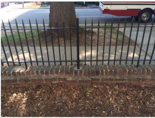
(265), Sumter Street - Campus Elevation Partial height wall with metal fence. Multiple repointing required. Cap work required. Metal to mortar connection needs work.
