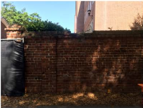
(67), Sumter Street - Street Elevation Full height wall with pier. Cap repair required.
