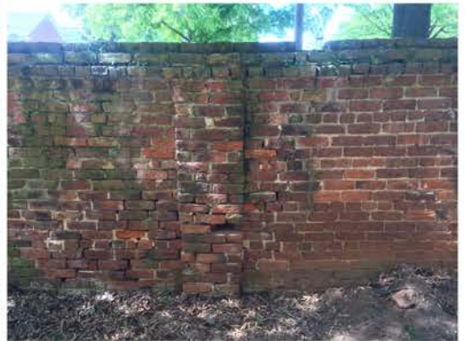
(309), Pendleton Street - Campus Elevation Full wall height with pier. Major repointing required. Multiple mortars.
