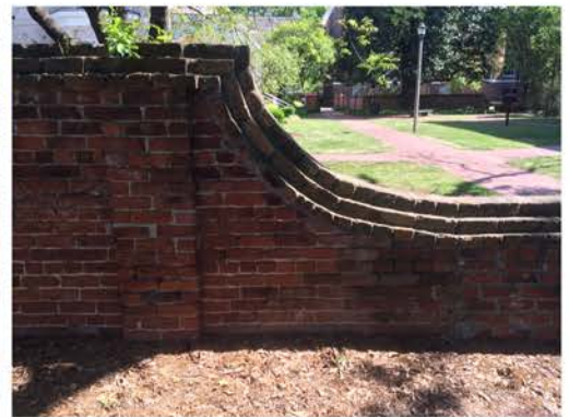
(180), Pendleton Street - Street Elevation Low wall to full height wall requiring brick and mortar replacement.
