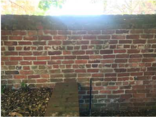
(256), Sumter Street - Campus Elevation Full height wall with partial height wall. Multiple repointing required. Cap work required.
