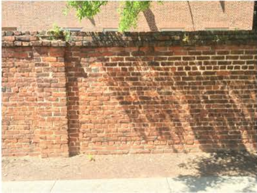
(40), Greene Street - Street Elevation Full height wall. Vegetation issues. Cap repair.
