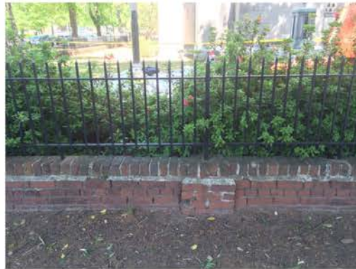
(152), Sumter Street - Street Elevation Low wall with fence. Mortar and cap replacement required. Multiple repointing required.
