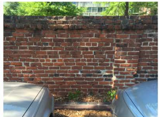
(288), Pendleton Street - Campus Elevation Full height wall with pier. Repointing required. Vegetation issues. Multiple mortars.
