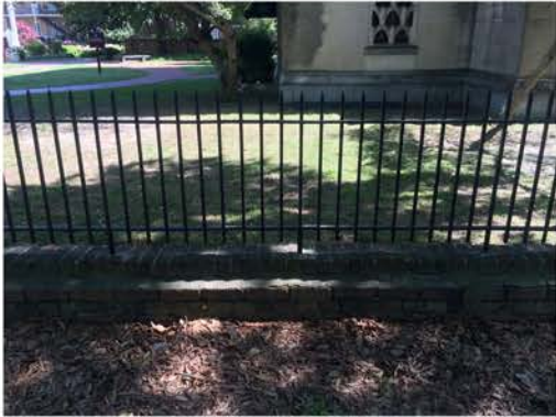
(172), Pendleton Street - Street Elevation Low wall with fence. Multiple repointing issues.
