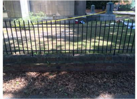
(162), Pendleton Street - Street Elevation Low wall with fence. Multiple repointing issues.
