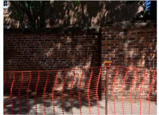
(54), Sumter Street - Street Elevation Full height wall. Repair cap. Large tree in background.
