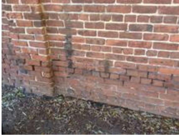
Lower Courses of Wall by Sumter near Pendleton (Note mortar recession in lower wall.)
