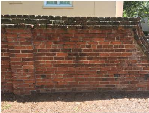
(199), Pendleton Street - Street Elevation Full height wall with pier. Multiple mortar repointing required.
