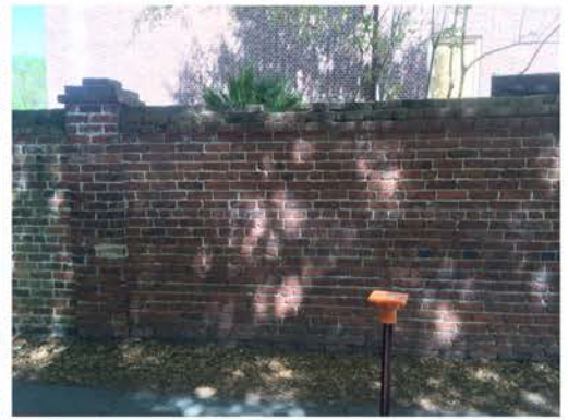
(63), Sumter Street - Street Elevation Full height wall with pier. Cap repair. Vegetation issues.
