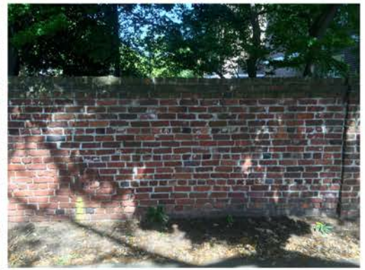
(135), Sumter Street - Street Elevation Full height wall with small pier. Incorrect mortar replacement.
