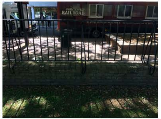
(231), Sumter Street - Campus Elevation Partial height wall with vertical rail. Vegetation issues typ.
