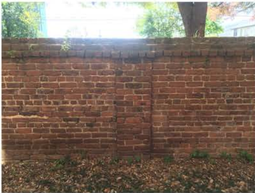
(247), Sumter Street - Campus Elevation Full height wall. Multiple repointing required. Vegetation issues.
