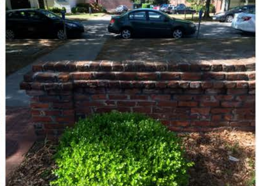
(282), Pendleton Street - Campus Elevation Partial height wall. Repointing required.
