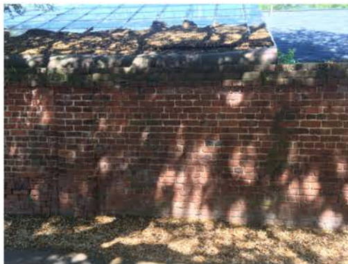
(71), Sumter Street - Street Elevation Full height wall with single pier. Cap repair required. Vegetation issues.
