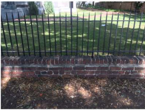
(145), Sumter Street - Street Elevation Low wall with fence. Mortar and cap replacement required.
