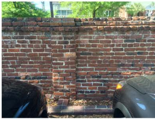
(290), Pendleton Street - Campus Elevation Full height wall with pier. Repointing required. Multiple mortars.
