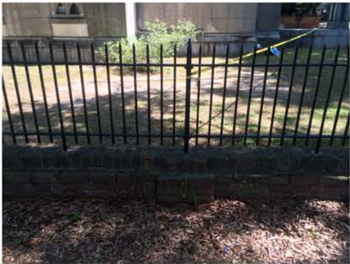
(163), Pendleton Street - Street Elevation Low wall with fence and pier. Multiple repointing issues.
