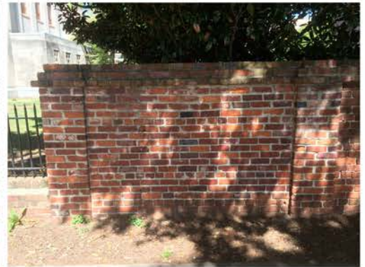
(141), Sumter Street - Street Elevation Full height wall with small pier. Multiple mortar replacement.
