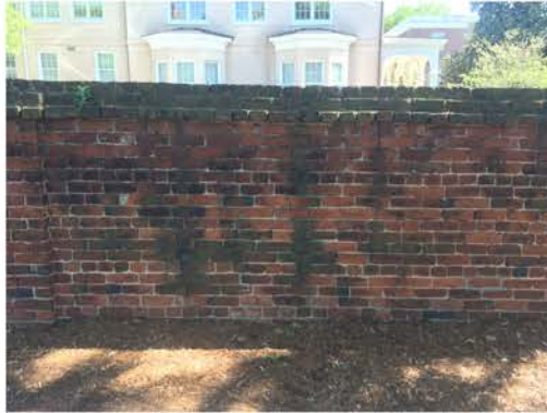
(185), Pendleton Street - Street Elevation Full height wall with pier. Cap and vegetation issues.
