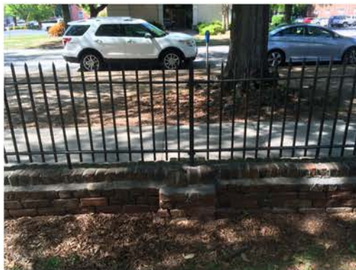
(275), Pendleton Street - Campus Elevation Low wall with fence and pier. Multiple repointing issues. Cap mortar issue.
