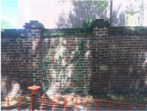
(64), Sumter Street - Street Elevation Full height wall with 2 piers. Cap repair. Repointing required between piers.
