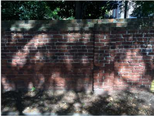
(136), Sumter Street - Street Elevation Full height wall with small pier. Incorrect mortar replacement.
