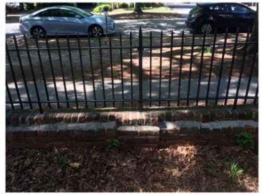
(279), Pendleton Street - Campus Elevation Low wall with fence and pier. Multiple repointing issues. Cap mortar issue.
