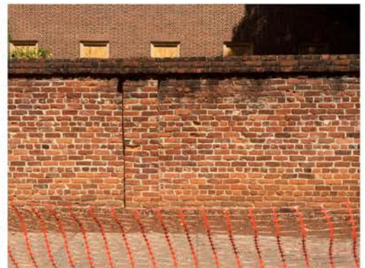
(60), Sumter Street - Street Elevation Full height wall with pier. Multiple face brick cracking.
