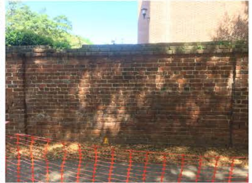
(66), Sumter Street - Street Elevation Full height wall with two piers. Cap repair required. Vegetation issues.
