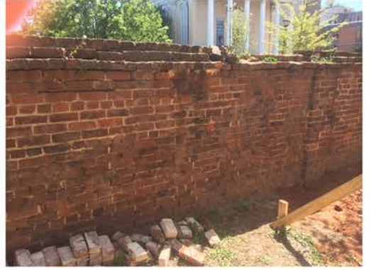
(6), Greene Street - Campus Elevation Full height wall. Cap replacement and repair required.
