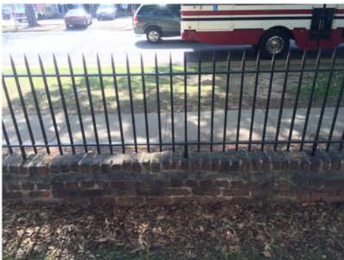
(262), Sumter Street - Campus Elevation Partial height wall with metal fence. Multiple repointing required. Cap work required.
