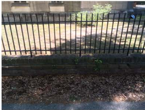
(164), Pendleton Street - Street Elevation Low wall with fence. Multiple repointing issues.
