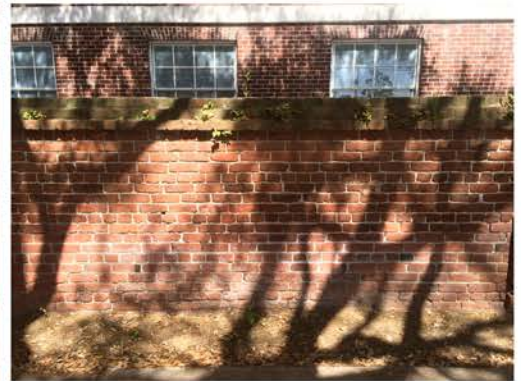
(129), Sumter Street - Street Elevation Full height wall. Vegetation issues.
