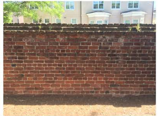
(189), Pendleton Street - Street Elevation Full height wall. Cap and vegetation issues.
