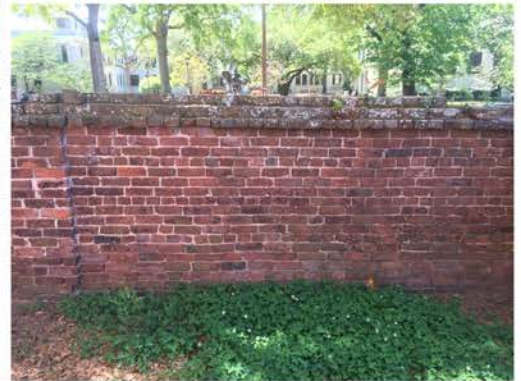
(33), Sumter Street - Campus Elevation Full height wall. Cap repair required.
