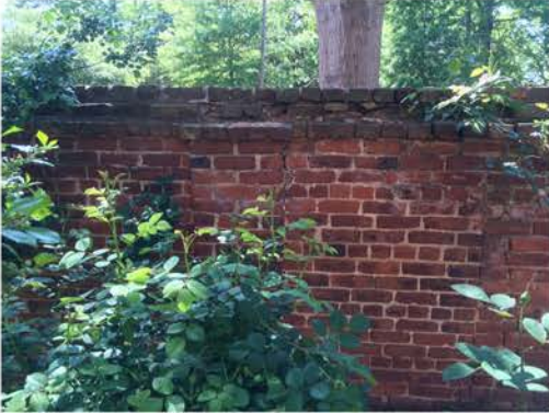
(88), Sumter Street - Campus Elevation Full height wall. Vertical cracks at pier.
