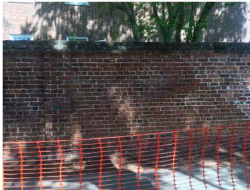
(56), Sumter Street - Street Elevation Full height wall. Multiple repointing issues.
