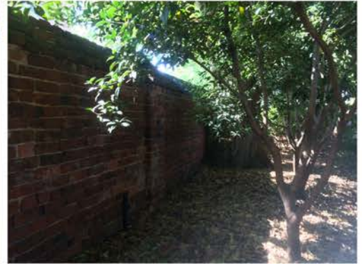
(258), Sumter Street - Campus Elevation Full height wall. Multiple repointing required. Large tree.
