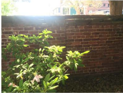
(257), Sumter Street - Campus Elevation Full height wall with pier. Multiple repointing required. Cap work required.
