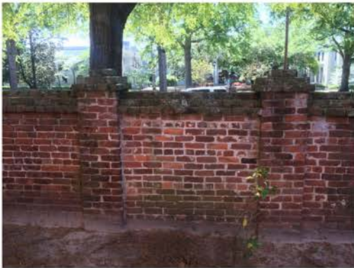
(31), Sumter Street - Campus Elevation Full height wall. Evaluate differ mortars in area between piers.
