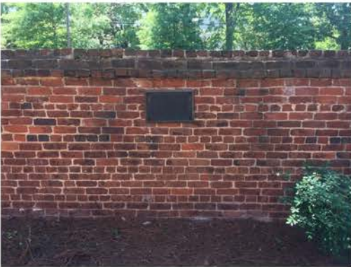
(91), Sumter Street - Campus Elevation Full height wall. Cap repair required. Sign in wall.
