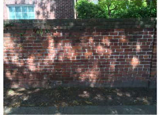
(126), Sumter Street - Street Elevation Full height wall with small pier. Vegetation issues.
