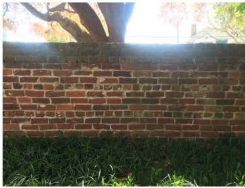
(254), Sumter Street - Campus Elevation Full height wall. Multiple repointing required. Cap work required.
