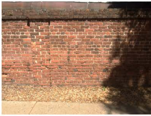
(74), Sumter Street - Street Elevation Full height wall with single pier. Multiple mortar and repointing issues. Vegetation issues at cap.
