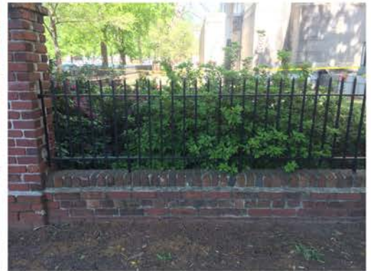
(153), Sumter Street - Street Elevation Low wall with fence transition to large corner. Mortar and cap replacement required. Multiple repointing required.
