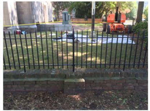
(159), Pendleton Street - Street Elevation Low wall with fence and pier. Mortar and cap replacement required.
