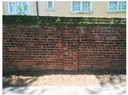
(207), Pendleton Street - Street Elevation Full height wall with pier. Multiple mortar repointing required. Cap replacement. Vegetation issues.
