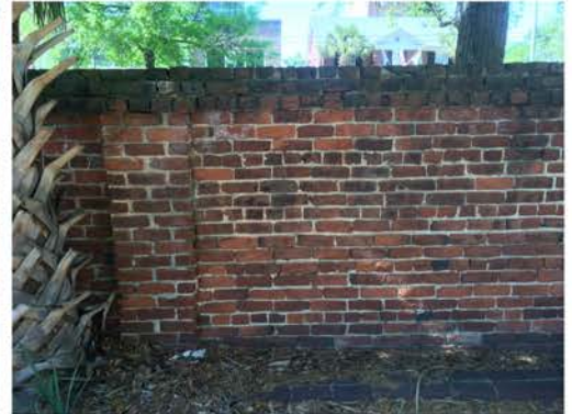
(294), Pendleton Street - Campus Elevation Full height wall with pier. Repointing required. Multiple mortars. Cap work required.
