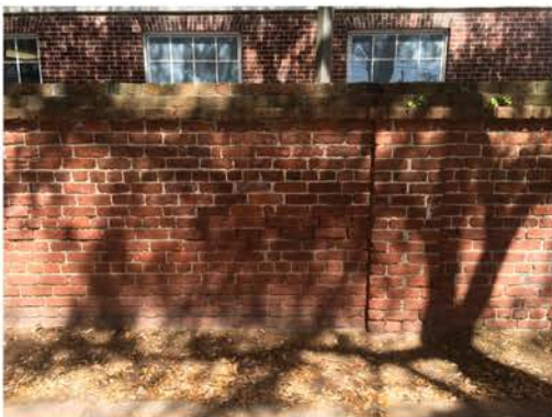
(130), Sumter Street - Street Elevation Full height wall with small pier. Vegetation issues. Repointing required at multiple areas.
