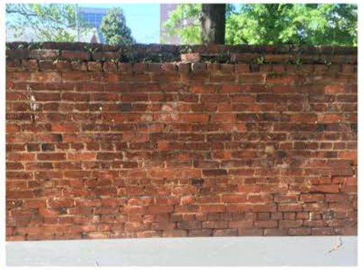
(303), Pendleton Street - Campus Elevation Full wall height. Repointing required. Multiple mortars. Vegetation issues.
