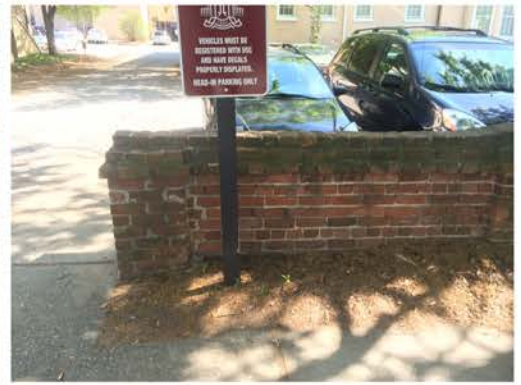
(195), Pendleton Street - Street Elevation Low wall height with piers. Cap and vegetation issues. Vertical cracking.
