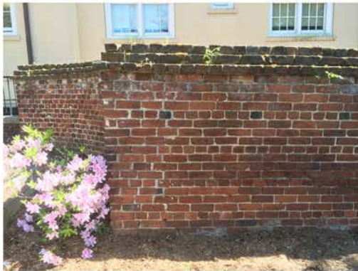
(212), Pendleton Street - Street Elevation Full height wall with pier to curving wall. Multiple mortar repointing required. Visible cracking.
