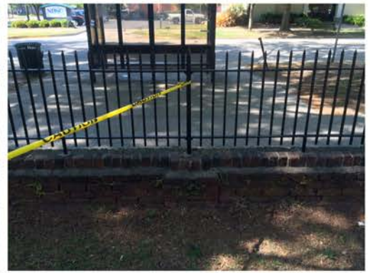
(267), Pendleton Street - Campus Elevation Low wall with fence and pier. Multiple repointing issues. Vegetation issues.
