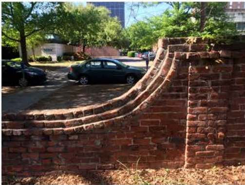
(283), Pendleton Street - Campus Elevation Patial height wall to full height wall with pier. Repointing required. Vegetation issues.
