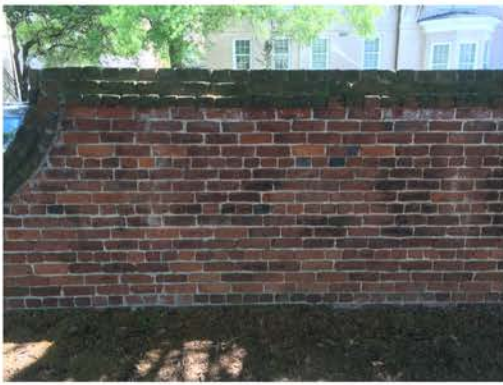
(193), Pendleton Street - Street Elevation Full height wall with pier. Cap and vegetation issues. Multiple mortar repointing required.
