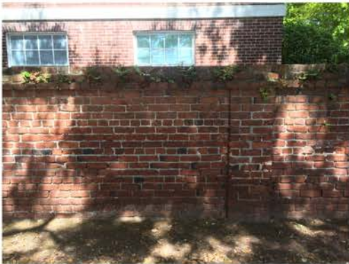
(127), Sumter Street - Street Elevation Full height wall with small pier. Multiple vegetation issues.
