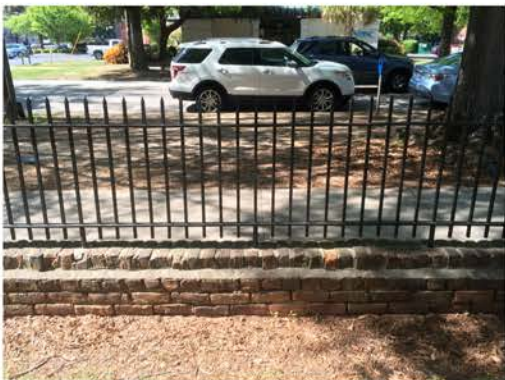
(274), Pendleton Street - Campus Elevation Low wall with fence. Multiple repointing issues. Vegetation issues. Cap mortar issue.
