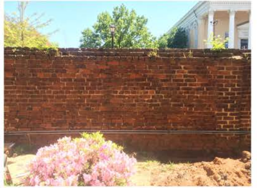
(12), Greene Street - Campus Elevation Full height wall. Repointing and vegetation removal required. Existing conduit removal required.
