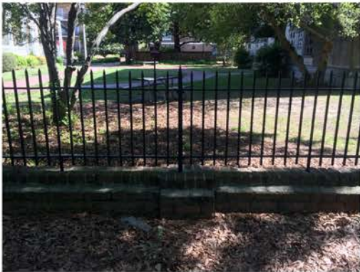
(175), Pendleton Street - Street Elevation Low wall with fence and pier. Multiple repointing issues.
