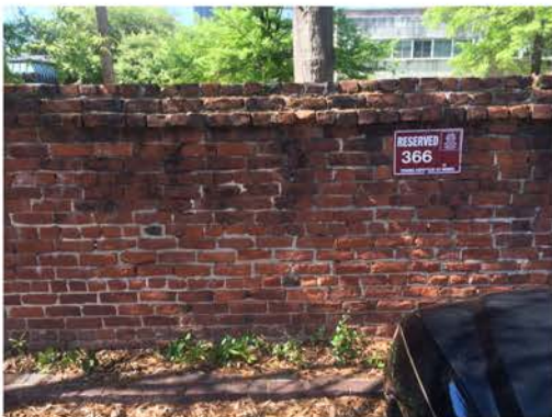
(286), Pendleton Street - Campus Elevation Full height wall with pier. Repointing required. Vegetation issues. Multiple mortars.
