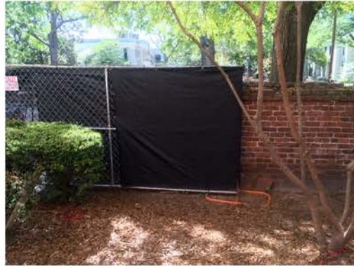
(29), Sumter Street - Campus Elevation Full height wall. Cap repair required.
