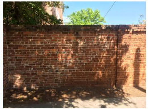
(51), Sumter Street - Street Elevation Full height wall. Multiple repointing issues.
