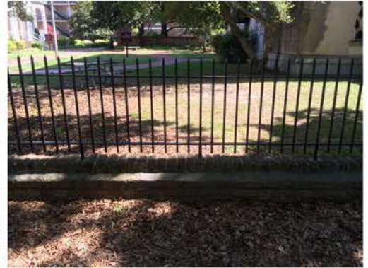
(174), Pendleton Street - Street Elevation Low wall with fence. Multiple repointing issues.
