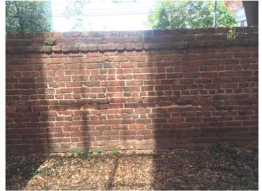
(246), Sumter Street - Campus Elevation Full height wall. Multiple repointing required. Vegetation issues.
