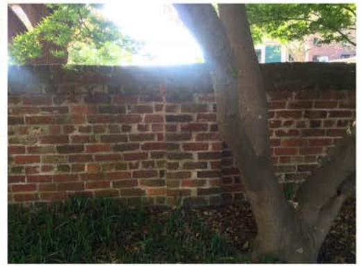
(255), Sumter Street - Campus Elevation Full height wall with pier. Multiple repointing required. Cap work required.
