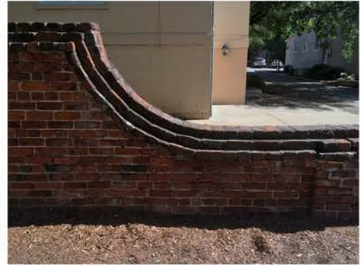
(198), Pendleton Street - Street Elevation Full height to partial height wall with pier. Multiple mortar repointing required.
