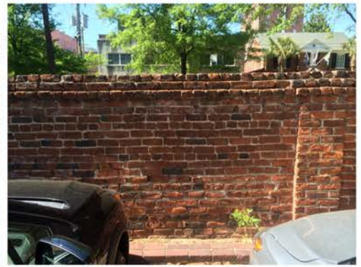
(291), Pendleton Street - Campus Elevation Full height wall with pier. Repointing required. Multiple mortars.
