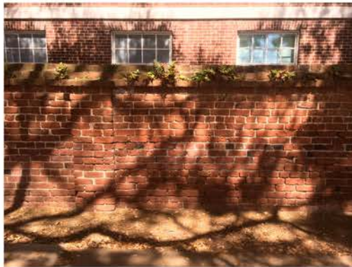
(128), Sumter Street - Street Elevation Full height wall with small pier. Vegetation issues.
