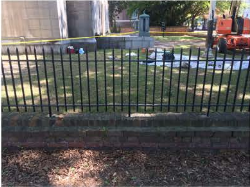
(160), Pendleton Street - Street Elevation Low wall with fence and pier. Multiple repointing issues.
