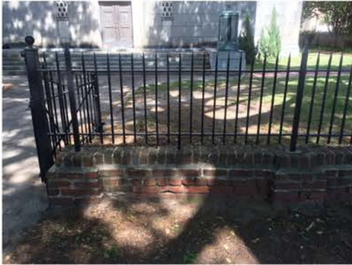
(148), Sumter Street - Street Elevation Low wall with fence and gate. Mortar and cap replacement required.
