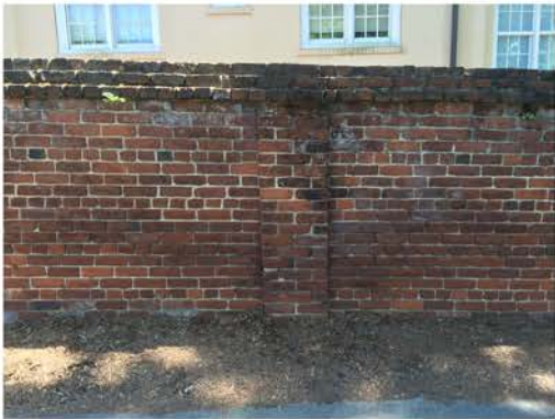
(211), Pendleton Street - Street Elevation Full height wall with pier. Multiple mortar repointing required. Cap replacement. Vegetation issues.
