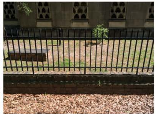
(168), Pendleton Street - Street Elevation Low wall with fence. Multiple repointing issues.
