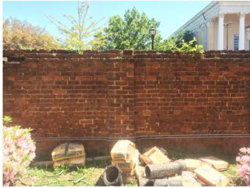
(11), Greene Street - Campus Elevation Full height wall. Repointing and vegetation removal required. Existing conduit removal required.
