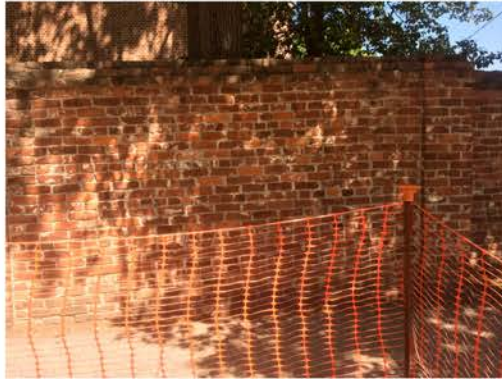
(53), Sumter Street - Street Elevation Full height wall. Brick bump out. Multiple repointing issues.
