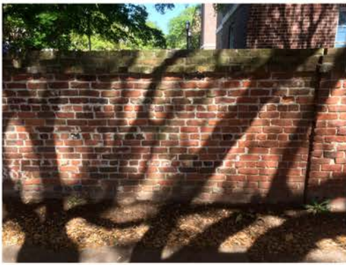
(133), Sumter Street - Street Elevation Full height wall with small pier. Incorrect mortar replacement.
