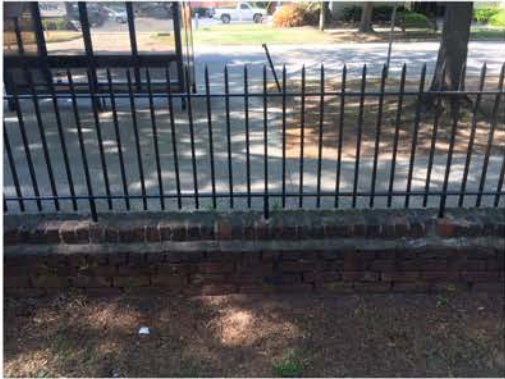
(268), Pendleton Street - Campus Elevation Low wall with fence. Multiple repointing issues. Vegetation issues.
