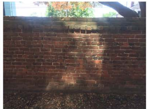
(252), Sumter Street - Campus Elevation Full height wall. Multiple repointing required. Cap work required.
