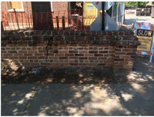
(37), Greene Street - Street Elevation Partial height wall with major vertical crack.
