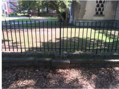
(173), Pendleton Street - Street Elevation Low wall with fence and pier. Multiple repointing issues.
