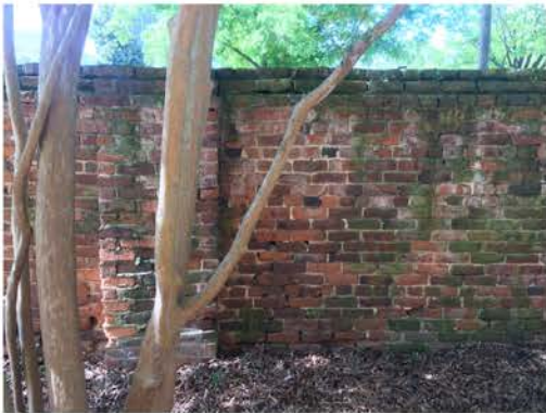
(307), Pendleton Street - Campus Elevation Full wall height with pier. Repointing required. Multiple mortars.
