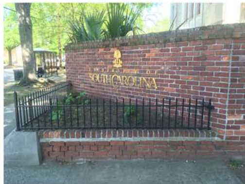
(155), Sumter Street - Street Elevation Large diagonal corner wall with small partial height wall and fence.. Mortar and cap replacement required. Multiple repointing and brick repair required.
