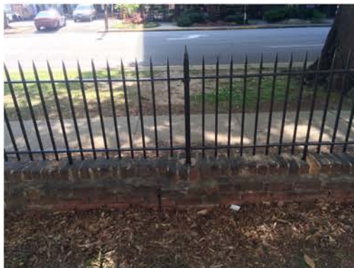
(263), Sumter Street - Campus Elevation Partial height wall with metal fence. Multiple repointing required. Cap work required. Metal to mortar connection needs work.
