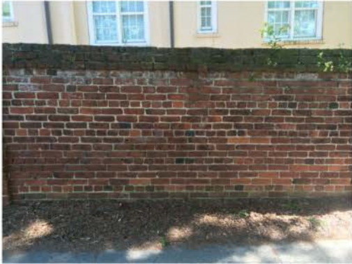
(208), Pendleton Street - Street Elevation Full height wall. Multiple mortar repointing required. Cap replacement. Vegetation issues.
