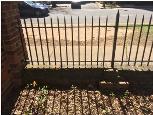
(259), Sumter Street - Campus Elevation Partial height wall with metal fence. Multiple repointing required.
