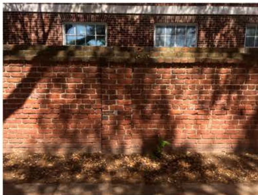
(131), Sumter Street - Street Elevation Full height wall with small pier. Vegetation issues. Repointing required at multiple areas.
