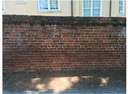
(210), Pendleton Street - Street Elevation Full height wall with pier. Multiple mortar repointing required. Cap replacement. Vegetation issues.
