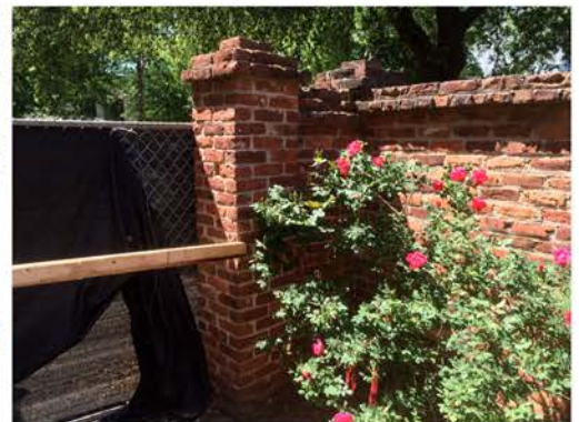
(36), Sumter Street - Campus Elevation Entry with full height wall and adjacent wall attached to pier. Cap repair required.
