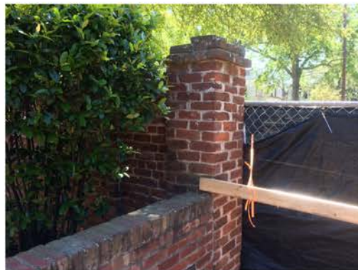
(35), Sumter Street - Campus Elevation Entry with full height wall and adjacent wall. Cap to be repaired.
