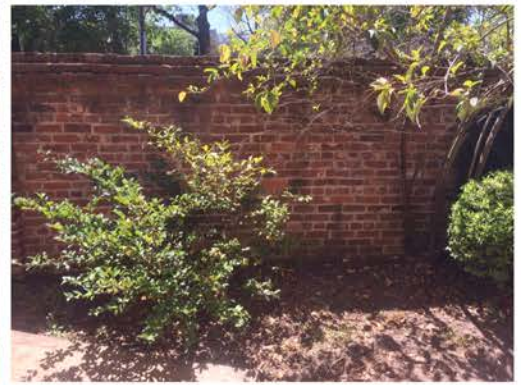
(27), Sumter Street - Campus Elevation Full height wall. Close vegetation removal required.
