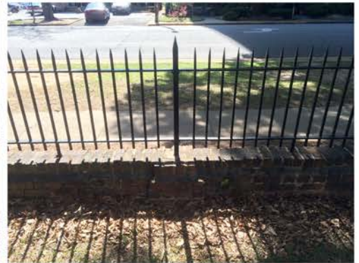
(261), Sumter Street - Campus Elevation Partial height wall with metal fence. Multiple repointing required. Cap work required.
