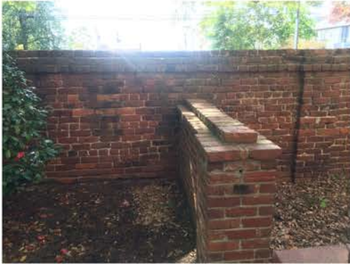
(244), Sumter Street - Campus Elevation Full height wall to partial height wall. Multiple repointing required.
