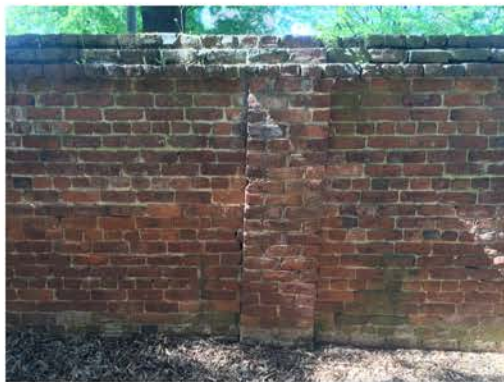
(311), Pendleton Street - Campus Elevation Full wall height with pier. Major repointing required. Multiple mortars.
