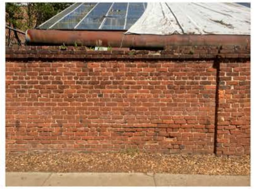
(75), Sumter Street - Street Elevation Full height wall with single pier. Multiple mortar and repointing issues. Cap repair required.
