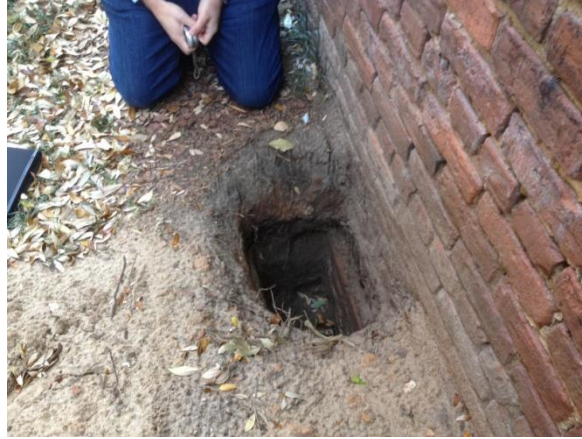
Excavation on Carolina Library on Sumter – Near location for Sumter 1 and Sumter 2
