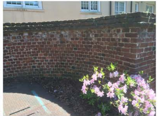
(213), Pendleton Street - Street Elevation Full height curved wall. Multiple mortar repointing required. Cap replacement. Vegetation issues.
