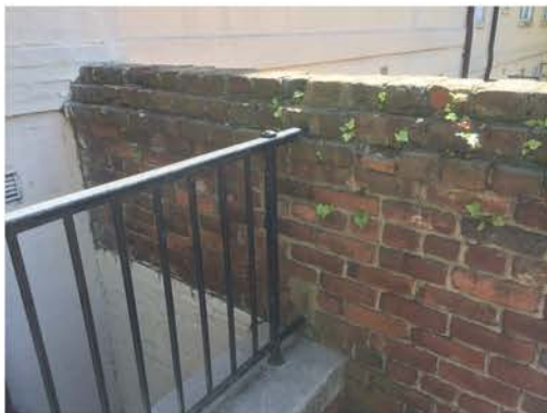
(215), Pendleton Street - Street Elevation Full height wall with rail. Multiple mortar repointing required. Wall to masonry building connection.
