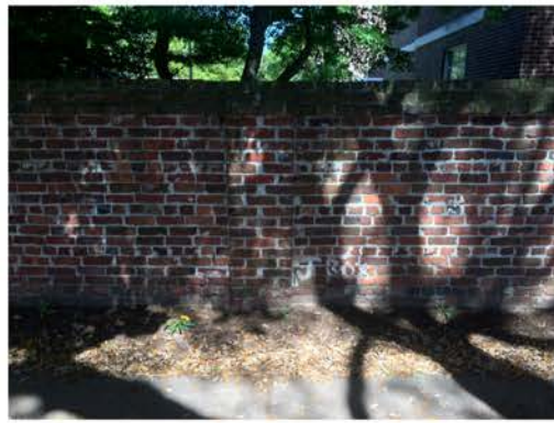
(134), Sumter Street - Street Elevation Full height wall with small pier. Incorrect mortar replacement.
