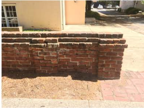
(197), Pendleton Street - Street Elevation Low wall height with piers. Cap and vegetation issues. Vertical cracking.
