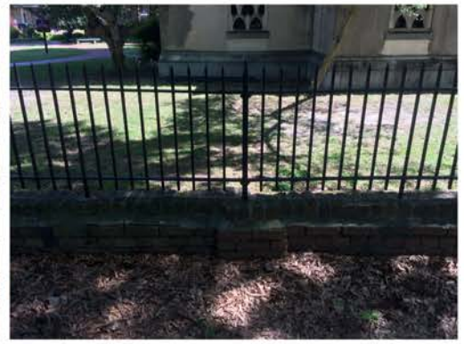
(171), Pendleton Street - Street Elevation Low wall with fence and pier. Multiple repointing issues.
