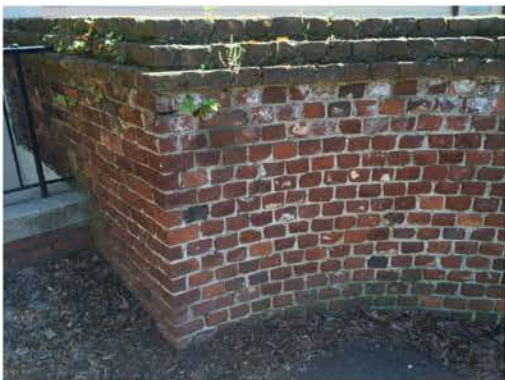
(214), Pendleton Street - Street Elevation Full height curved wall. Multiple mortar repointing required. Cap replacement. Vegetation issues.
