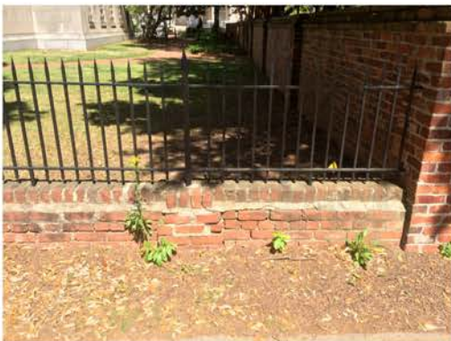
(142), Sumter Street - Street Elevation Low wall with fence. Brick repair/replacement required. Mortar replacement required.
