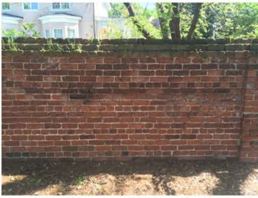
(181), Pendleton Street - Street Elevation Full height wall. Cap and vegetation issues.
