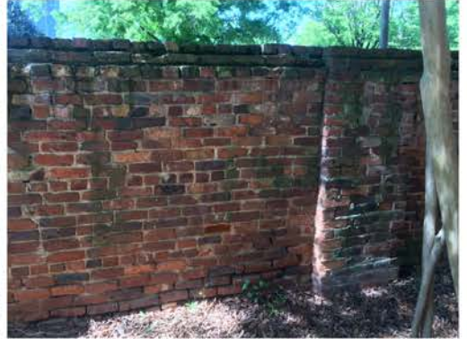
(306), Pendleton Street - Campus Elevation Full wall height. Repointing required. Multiple mortars.
