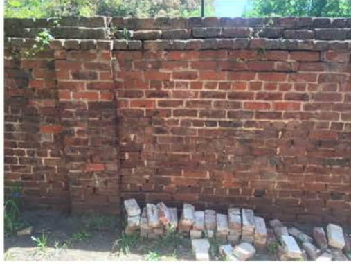
(5), Greene Street - Campus Elevation Full height wall. Repointing required typ.
