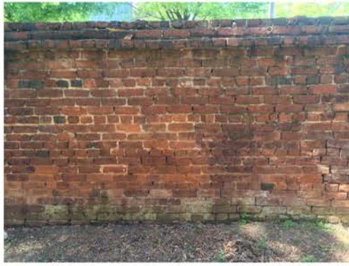
(314), Pendleton Street - Campus Elevation Full wall height. Major repointing required. Multiple mortars. Vertical cracking.
