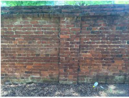
(313), Pendleton Street - Campus Elevation Full wall height with pier. Major repointing required. Multiple mortars. Vegetation issues.
