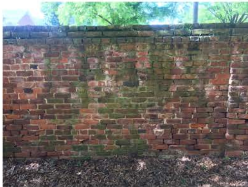
(308), Pendleton Street - Campus Elevation Full wall height. Major repointing required. Multiple mortars.
