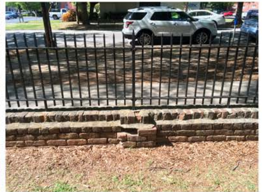
(273), Pendleton Street - Campus Elevation Low wall with fence and pier. Multiple repointing issues. Vegetation issues. Cap mortar issue.
