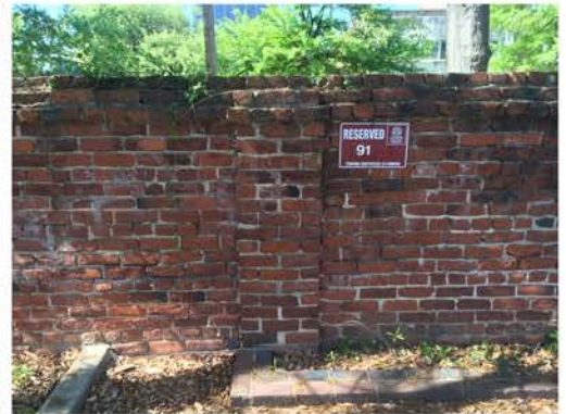
(285), Pendleton Street - Campus Elevation Full height wall with pier. Repointing required. Vegetation issues. Multiple masonry connections.
