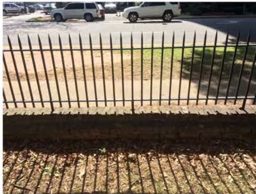
(260), Sumter Street - Campus Elevation Partial height wall with metal fence. Multiple repointing required. Cap work required.
