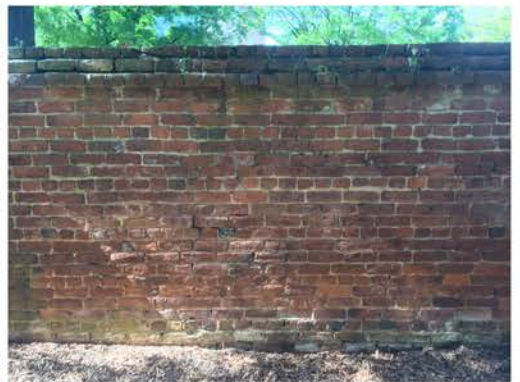
(312), Pendleton Street - Campus Elevation Full wall height. Major repointing required. Multiple mortars.
