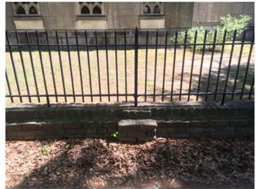
(165), Pendleton Street - Street Elevation Low wall with fence and pier. Multiple repointing issues.
