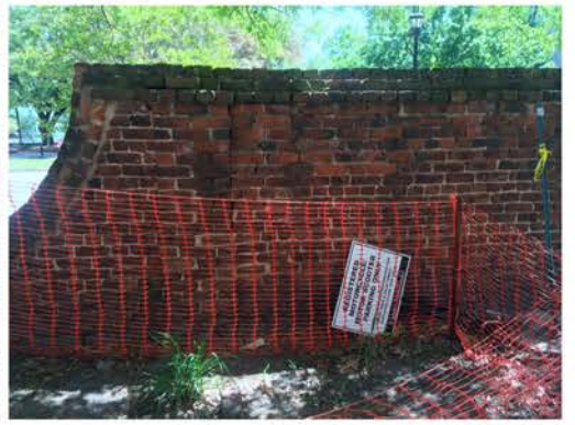
(3), Greene Street - Campus Elevation Full height wall transition with major diagonal crack.
