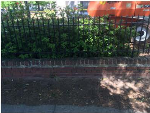
(151), Sumter Street - Street Elevation Low wall with fence. Mortar and cap replacement required. Multiple repointing required.
