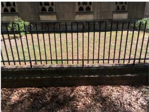
(166), Pendleton Street - Street Elevation Low wall with fence. Multiple repointing issues.
