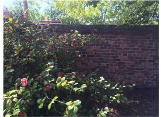
(18), Sumter Street - Campus Elevation Full height wall. Repointing required.
