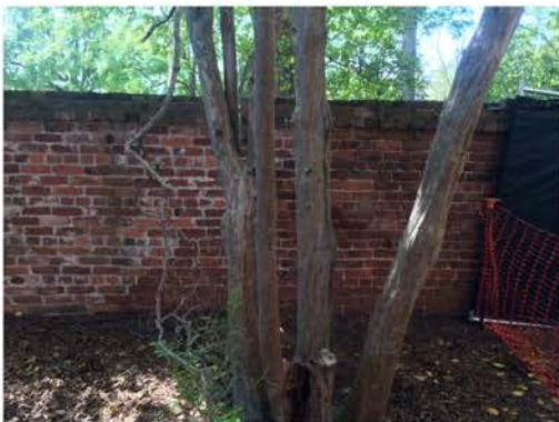
(22), Sumter Street - Campus Elevation Full height wall. Major mortar repointing.
