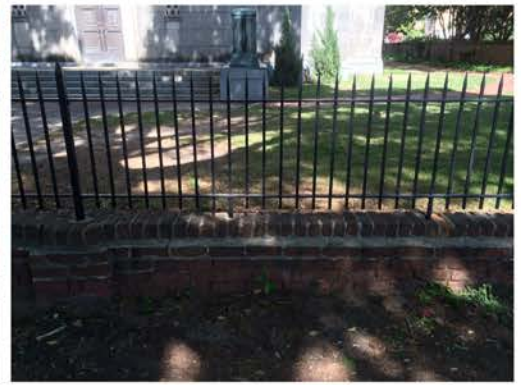
(147), Sumter Street - Street Elevation Low wall with fence. Mortar and cap replacement required.
