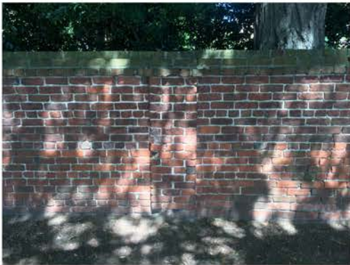
(139), Sumter Street - Street Elevation Full height wall with small pier. Incorrect mortar replacement. Visible cracking.
