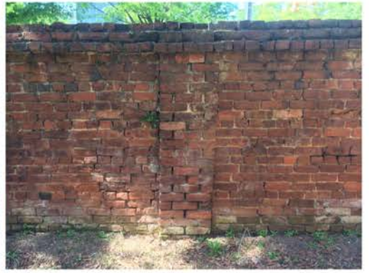
(315), Pendleton Street - Campus Elevation Full wall height with pier. Major repointing required. Multiple mortars.
