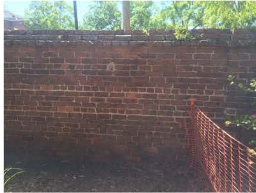
(17), Sumter Street - Campus Elevation Full height wall. Repointing required. Major vertical crack.
