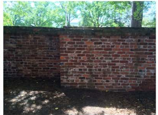
(21), Sumter Street - Campus Elevation Full height wall. Brick face and cap built up residue.
