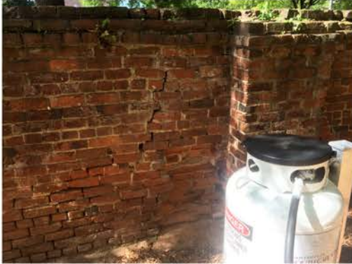
(304), Pendleton Street - Campus Elevation Full wall height. Repointing required. Multiple mortars. Visible cracking.
