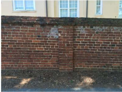
(209), Pendleton Street - Street Elevation Full height wall with pier. Multiple mortar repointing required. Cap replacement. Vegetation issues.
