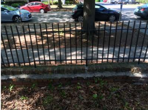
(280), Pendleton Street - Campus Elevation Low wall with fence and pier. Multiple repointing issues. Cap mortar issue very serious.
