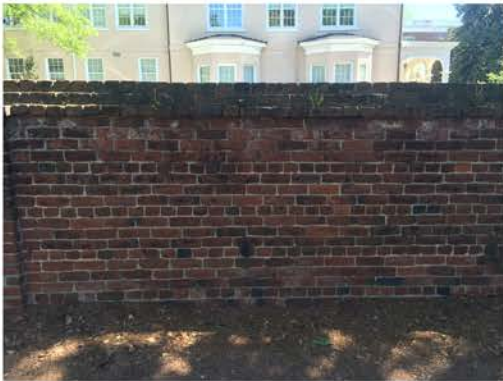
(187), Pendleton Street - Street Elevation Full height wall. Cap and vegetation issues.
