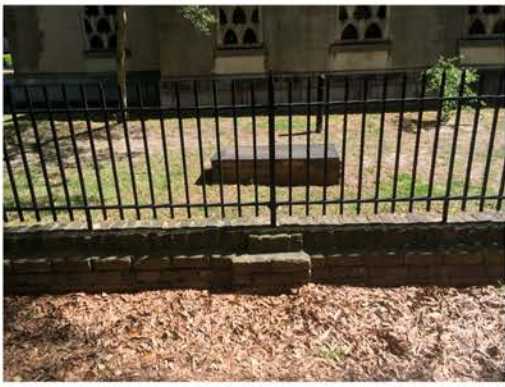
(169), Pendleton Street - Street Elevation Low wall with fence and pier. Multiple repointing issues.
