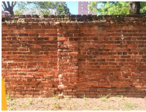
(302), Pendleton Street - Campus Elevation Full wall height with pier and multiple structural issues. Repointing required. Multiple mortars. Vegetation issues.
