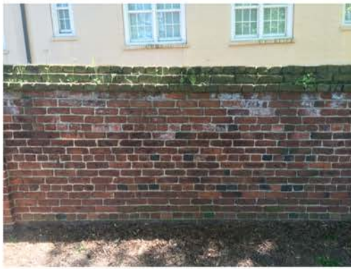
(206), Pendleton Street - Street Elevation Full height wall. Multiple mortar repointing required. Cap replacement. Vegetation issues.
