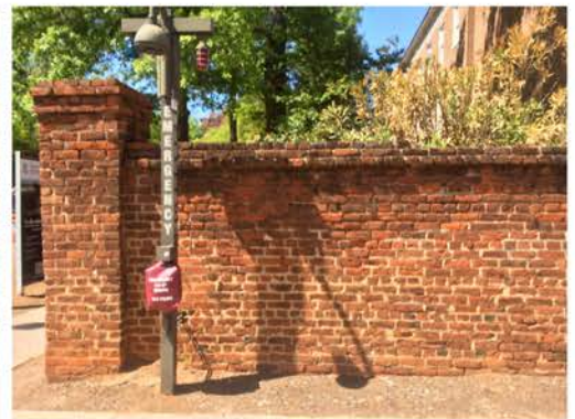
(48), Greene Street - Street Elevation Full height wall. Corner Pier. Cap repair issues.
