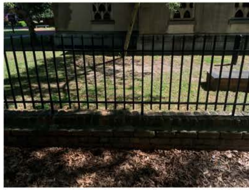
(170), Pendleton Street - Street Elevation Low wall with fence. Multiple repointing issues.
