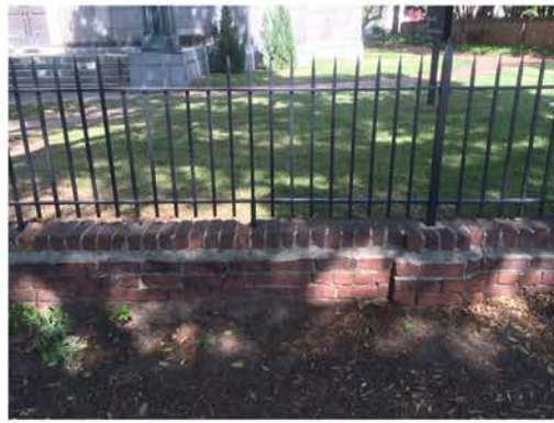
(146), Sumter Street - Street Elevation Low wall with fence. Mortar and cap replacement required. Brick replacement required.
