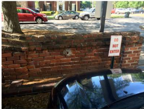
(296), Pendleton Street - Campus Elevation Partial wall height. Repeating required. Multiple mortars and missing brick.
