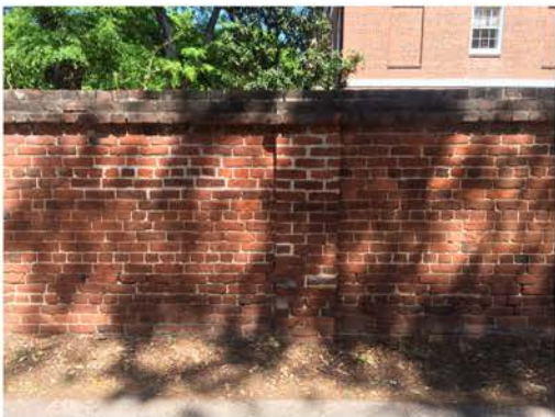
(82), Sumter Street - Street Elevation Full height wall. Multiple mortar and repointing issues.
