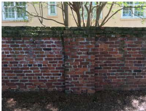
(203), Pendleton Street - Street Elevation Full height wall with pier. Multiple mortar repointing required. Cap replacement. Vegetation issues.
