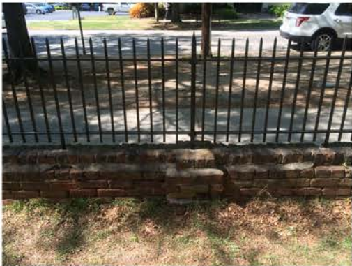
(271), Pendleton Street - Campus Elevation Low wall with fence and pier. Multiple repointing issues. Vegetation issues. Cap mortar issue. Visible cracking.
