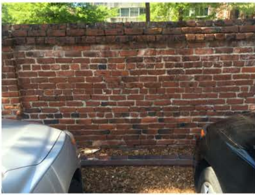
(289), Pendleton Street - Campus Elevation Full height wall with pier. Repointing required. Vegetation issues. Multiple mortars.
