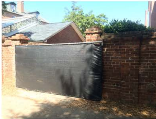
(68), Sumter Street - Street Elevation Full height wall with multiple entry piers. Cap repair required.
