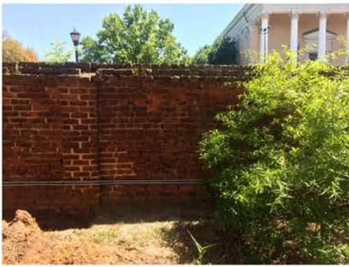
(13), Greene Street - Campus Elevation Full height wall. Repointing and vegetation removal required. Existing conduit removal required.
