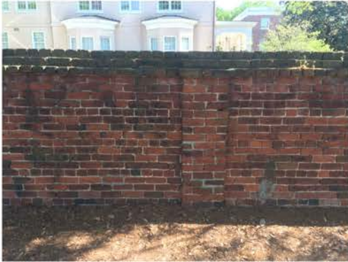
(184), Pendleton Street - Street Elevation Full height wall with pier. Cap and vegetation issues.
